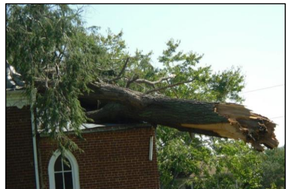
Figure 32- Christ Church (062-0003) was damaged by a September 2012 storm (photo courtesy: J.P. Harvey, nelsoncountylife.com)
