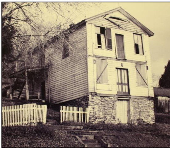
Figure 29- The Nelson Store (062-0218) burned in the early 1990s. Only its foundation remains.
